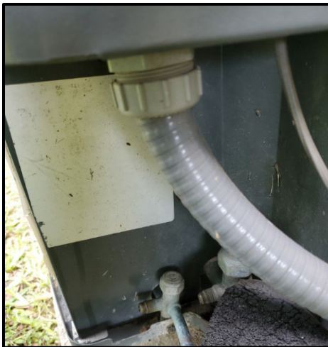
Outdoor unit nameplate unreadable
