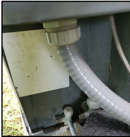
Outdoor unit nameplate unreadable
