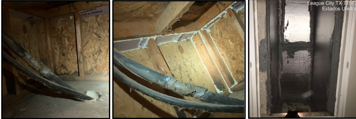
Supply air plenum before and after
