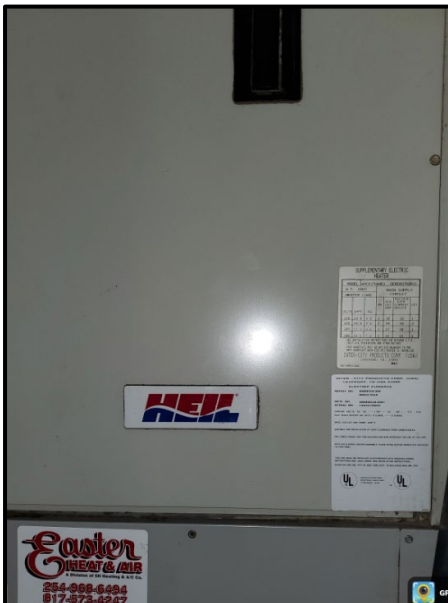
Indoor unit (electric resistance)
