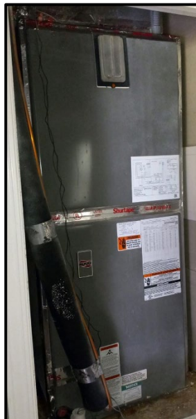
Indoor unit (electric resistance)
